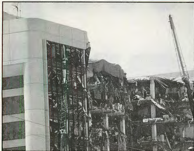
Skyline of A.P. Murrah Federal Building after bombing shows how blast went upward through 10 stories, inward the depth of several offices.
